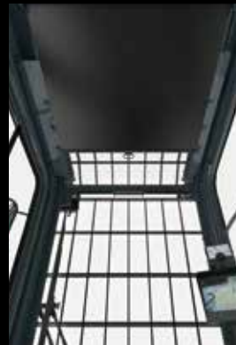
Sun screen for skylight
